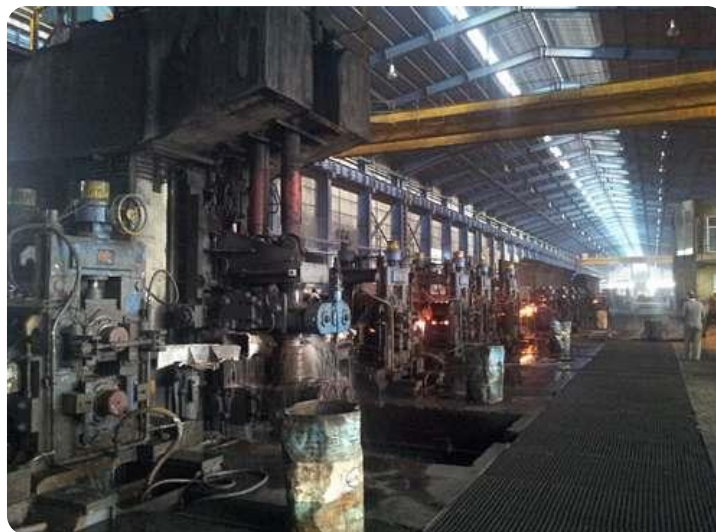
Rebars rolling mill stands
