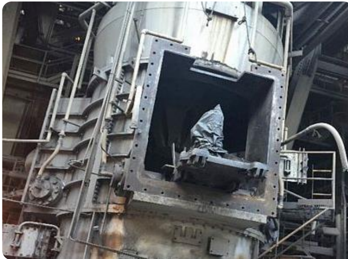
Coal grinding mill
