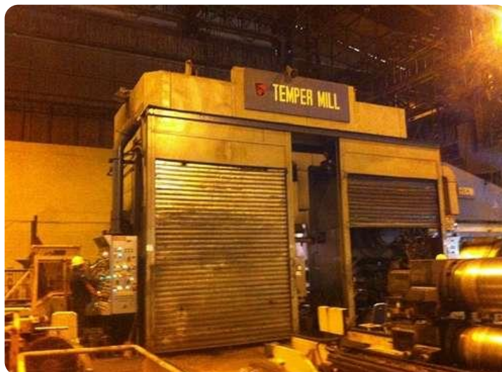
Cold rolling mill, temper mill line
