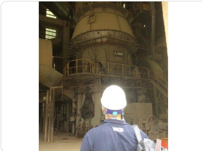
Vertical raw mill UBE
