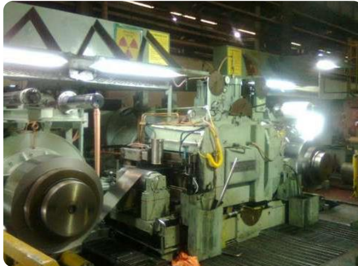
Cold rolling mill, skin pass mill
