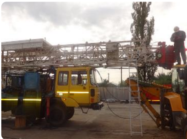
Pulley on a crane for oil equipment
