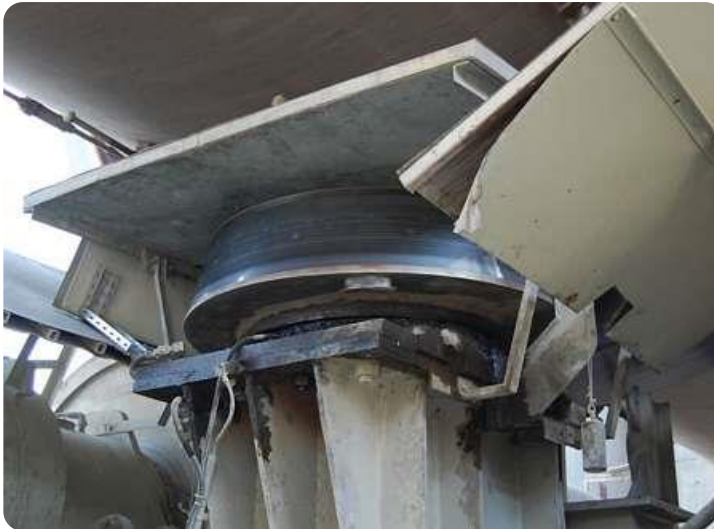
Rotary kiln equipment
