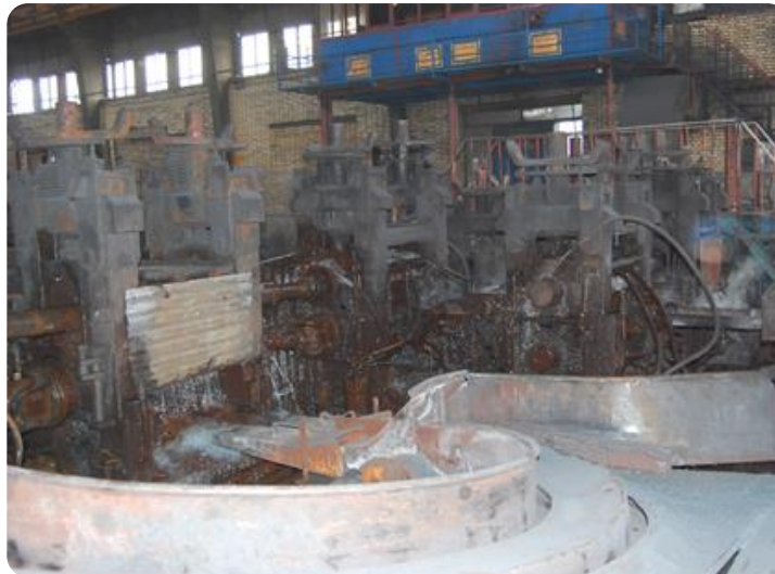
Rebars rolling mill
